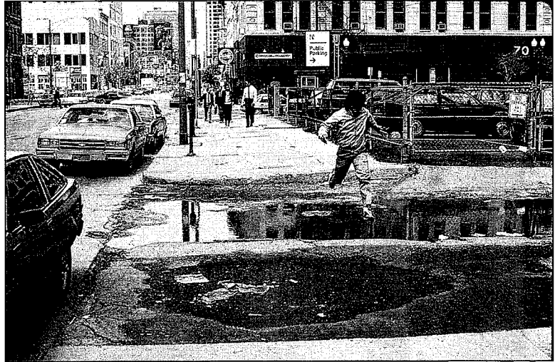
FIGURE 3-12. Poor drainage can adversely affect the usefulness of sidewalks.
