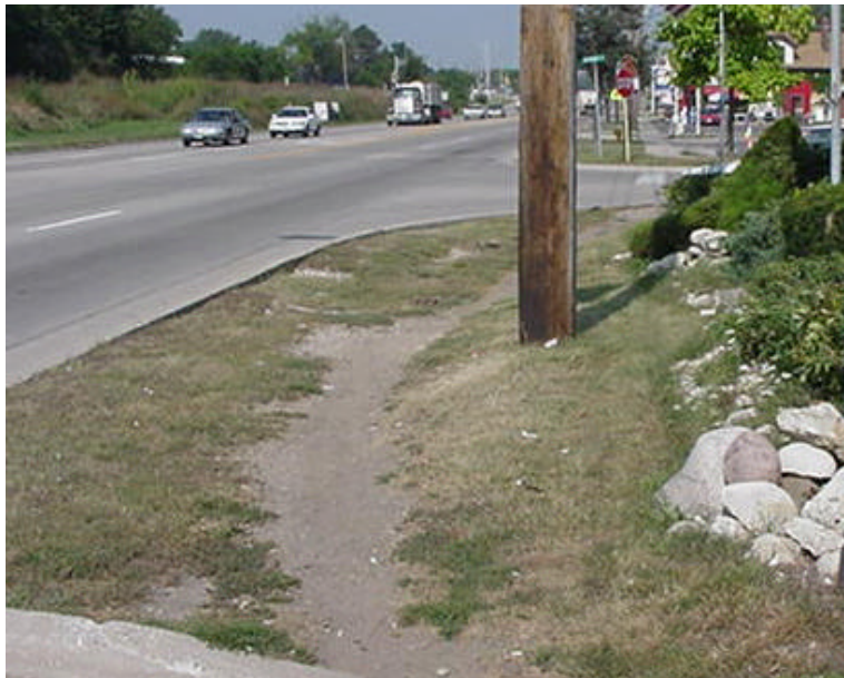
It is obvious that pedestrians use this area, due to the “desire lines.” Limited right-of-way and utilities will make retrofitting a sidewalk difficult along this arterial road.
