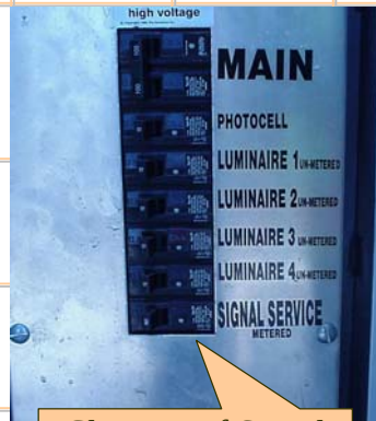
Close-up of Signal Service Cabinet
