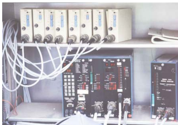
Figure 4-1. Controller, Detectors and Conflict Monitor in a Cabinet.
