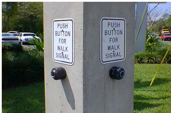
Figure 4-5. Typical Pedestrian Push-Button Detectors.
